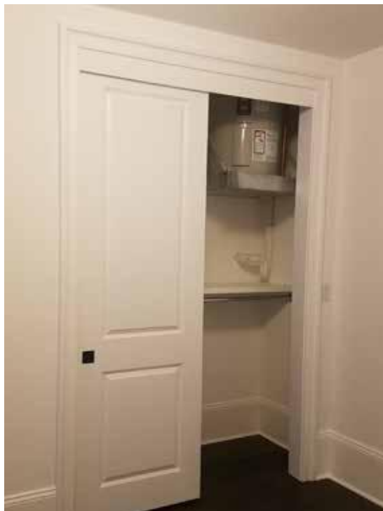
[43] Relocating mechanical equipment in interior spaces should be limited to utilitarian spaces like closets or mechanical rooms. Photo: Mary Lane Carleton
