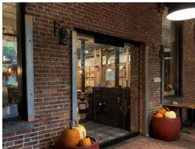
[25] Permanent stanchions at windows and doors in this former industrial mill in Baltimore, MD, are used to attach temporary floodgates to protect openings in the event of a flood. Depending on their size, color, and finish, these stanchions can be quite noticeable. In the case of an industrial property, this may not cause a significant change in historic character. In a different type of building, it is important to ensure that such permanent features blend in and are as visually unobtrusive as possible. Photo: Jennifer Parker/NPS
