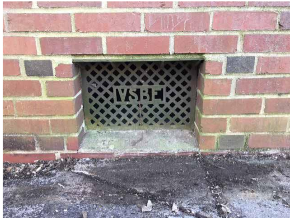
[56] To create a watertight seal around the building, any existing vents or openings below the established flood risk level must be sealed during a flood. Vents that cannot be sealed internally will require an exterior and/or interior cover to keep water from entering the building. Photo: Chelius Carter
