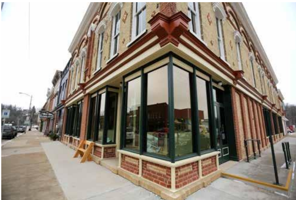
Figure 6: Exterior of the building after the dry floodproofing project is complete. The exterior steel storefront framing is a historic feature, painted green above the storefront and cream below after rehabilitation. Photo: Dave Kettering/Telegraph Herald
