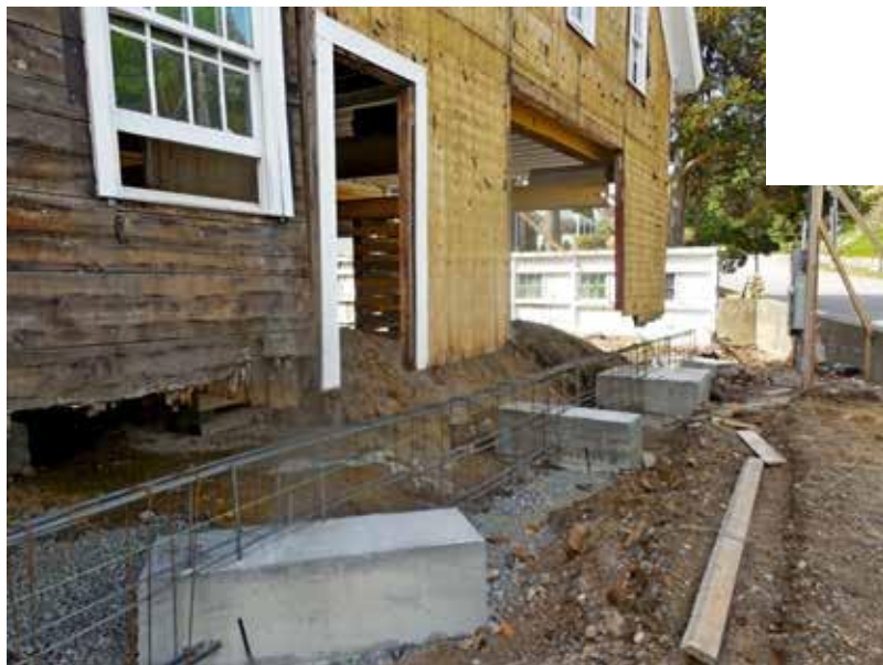
Figure 3: The structure was lifted in sections several feet in the air to provide space and access for foundation work. Photo: GNCB Consulting Engineers
