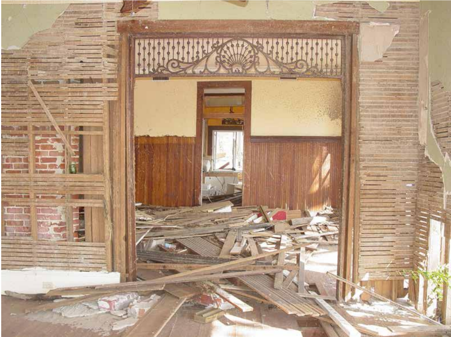
[6] Flood waters can also damage interior spaces. This historic home in Bay St. Louis, MS, was severely impacted by the storm surge from Hurricane Katrina. Even with such dramatic damage, it is crucial to properly assess the condition of historic materials and identify what remains and can be retained. In this case, most of the woodwork, the wood wainscot, upper sections of plaster in some rooms, and some areas of flooring were cleaned, dried, and repaired. Photo: Mississippi Department of Archives and History, Mississippi Historic Resources Inventory (HRI) Database. http://www.apps.mdah.ms.gov/Public
