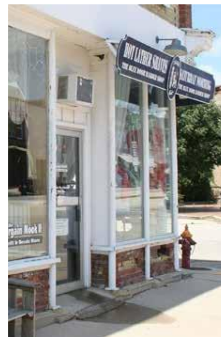
Figure 3: The historic storefronts and brick bulkhead were extant before floodproofing work began on the Driver Opera House. Photo: KONTEXT architects llc
