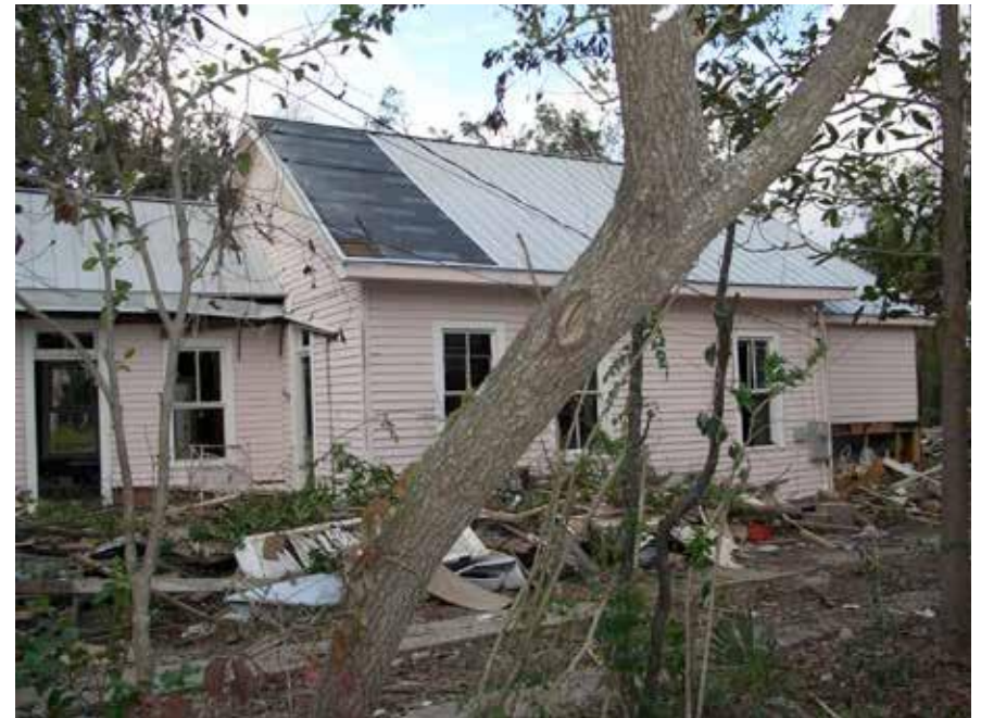
Figure 4: This photo of the hurricane damage shows that part of the roof was stripped away, and debris littered the site around the house. Photo: Mississippi Department of Archives and History, Mississippi Historic Resources Inventory (HRI) Database. http://www.apps.mdah.ms.gov/Public
