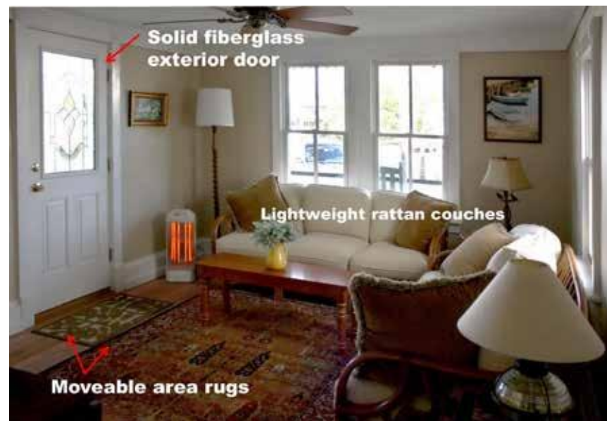
Figure 7: After repairs and wet floodproofing measures have been implemented, the new floor and wall surfaces are flood-damage resistant. The front door and windows were also replaced with more compatible designs using flood-damage resistant materials Photo: Mary Delaney Krugman, JD, MSHP
