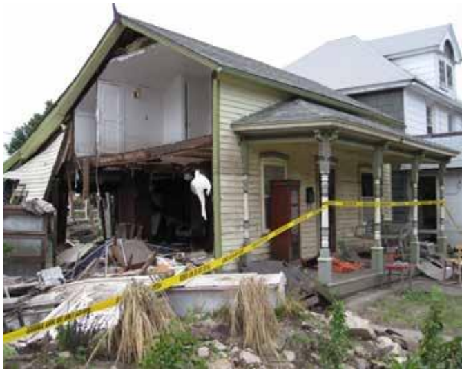
[8] Understanding the characteristics of a flood are critical to understanding property risk. Significant structural damage occurred to this building as a result of a riverine flood in Cedar Rapids, IA, in 2008. Photo: Greg Januska
