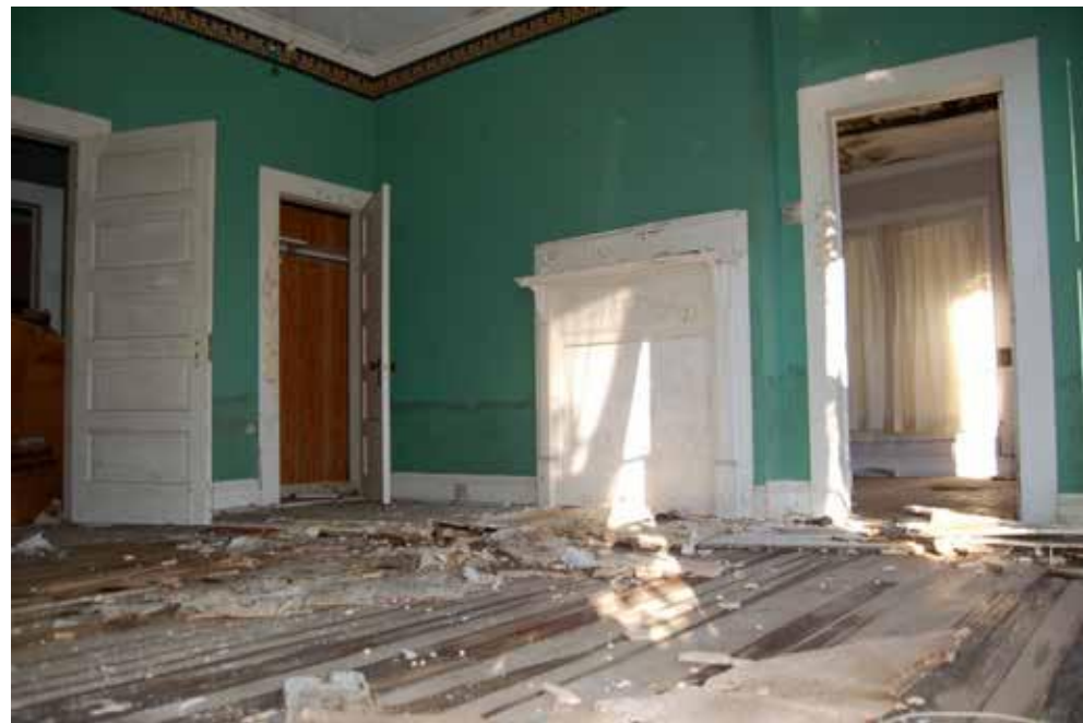
[59] Flood waters can have a significant impact on historic building interiors. Historic features and materials can often be retained and repaired and should not be preemptively removed or replaced. Much of the interior of this flooded historic property in Gulfport, MS, was able to be cleaned and retained.
