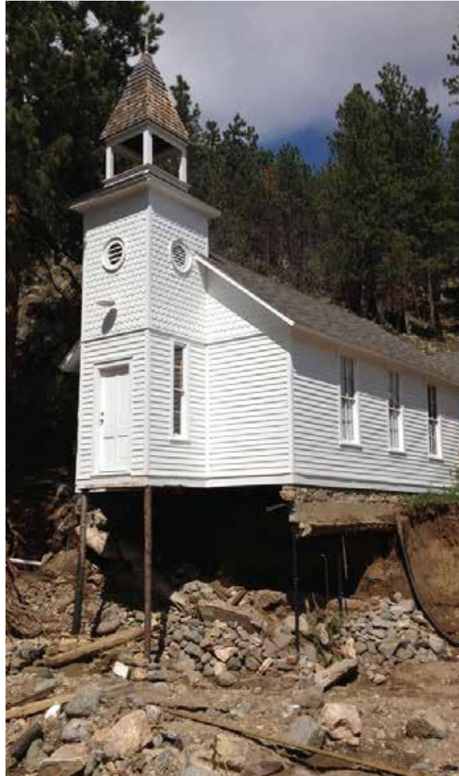
[9] Fast-moving flood waters can undermine a foundation or scour out land around a building. The Little Church of the Pines in Salina, CO, was left structurally compromised after heavy rains caused flooding in the Front Range of the Rocky Mountains in 2013. Photo: Burton Construction burton-construction.com
