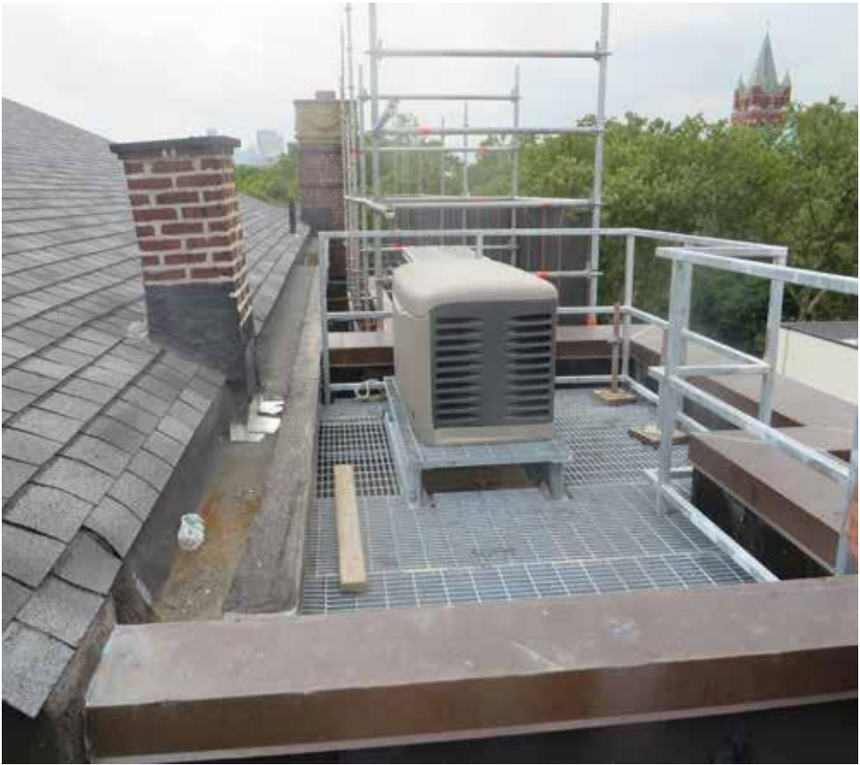
[46] For many buildings in flood-prone areas, having a generator on site may be a necessity to provide emergency power for pumps and other mechanical equipment. This public library in Hoboken, NJ, has a generator located on a flat roof high above any flood waters and not visible from the street. Photo: David V. Abramson for Hoboken Public Library
