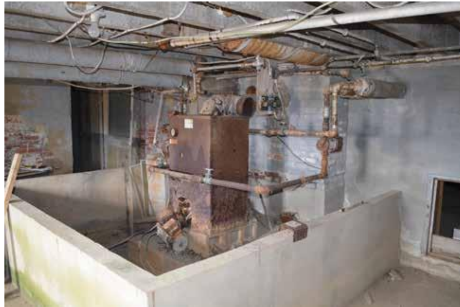
[42] Mechanical equipment that remains in a basement that is likely to flood should be enclosed behind waterproof walls. The walls may be partial height, as shown in this example, if flood waters are not expected to exceed that height. In other cases, waterproof enclosures must fully surround the equipment, which can be accessed by submarine-quality doors or hatches. Photo: Quinn Evans
