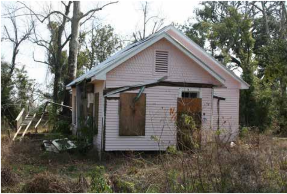
Figure 3: Hurricane Katrina destroyed the wrap-around front porch and knocked the house off the pier foundation. This photo was taken after the site had been cleared and windows and doors were temporarily boarded. Photo: Mississippi Department of Archives and History, Mississippi Historic Resources Inventory (HRI) Database. http://www.apps.mdah.ms.gov/Public
