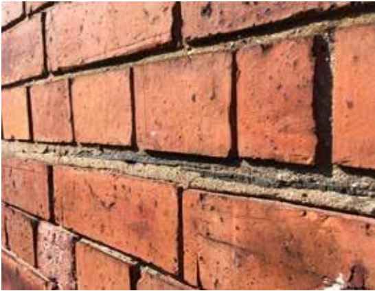
[66] In order to limit the absorption of flood waters, a horizontal waterstop joint can be installed in a building's walls depending upon the wall material and construction. This was also done historically, as shown in this historic brick wall with slate embedded in the mortar to limit water wicking up the wall. Photo: eagle/stock.adobe.com
