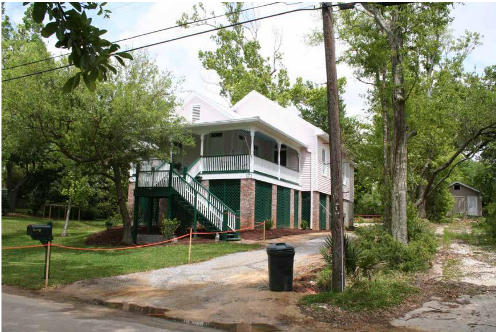
Figure 5: A taller foundation was constructed to elevate the house above the established flood risk level. While the house is higher than it was historically, the change is still in keeping with the historic character of the house, which had been on a tall foundation historically. The change is also consistent with historic regional traditions of adapting buildings to flood events. Additionally, the details of the foundation, with the brick piers and painted lattice, matches features of the historic design. The stairs access the porch in the historic location, but the extended run required by the taller foundation is turned 90 degrees below the landing to allow a surviving tree to remain in front of the house. A small retaining wall behind the tree holds fill that was added around the house to mask some of the change in height. Photo: Mississippi Department of Archives and History, Mississippi Historic Resources Inventory (HRI) Database. http://www.apps.mdah.ms.gov/Public
