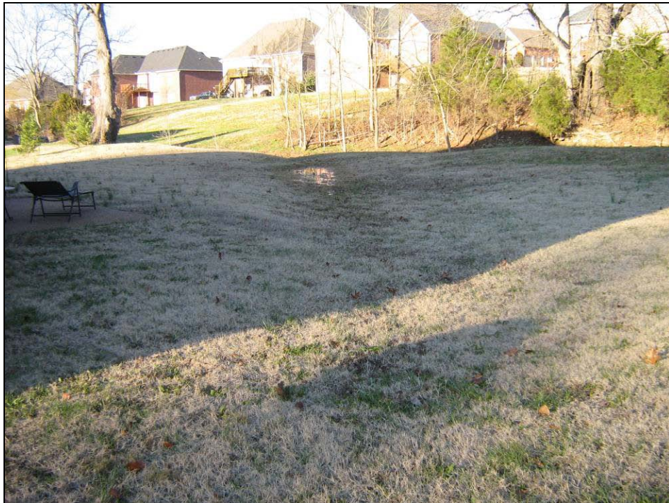
Item 4 - 413 Barnes Drive. Grade ditch to drain into creek. Note standing water. Looking downstream (east) from Barnes Dr. Picture 2350.
