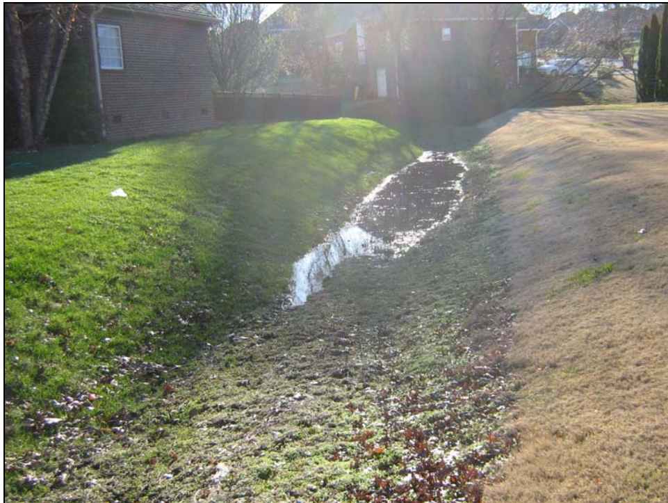
Item 8 – Looking west from Lexington Dr. cross drain (south of Letcher Ave). Grade ditch to drain into creek. Note standing water. Picture 2315.
