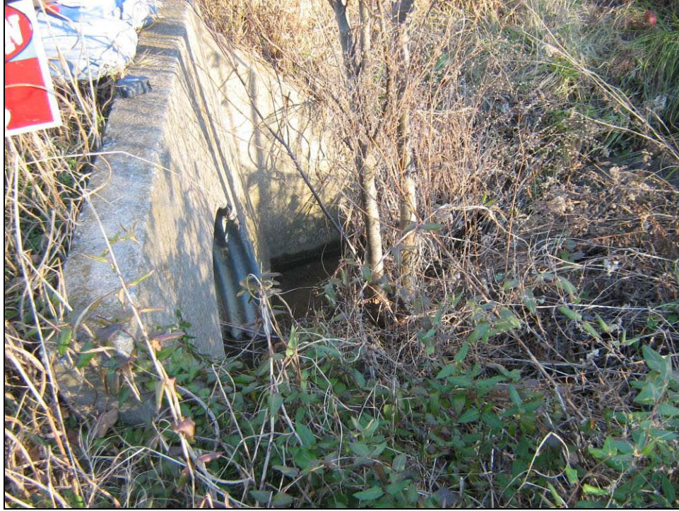
Item 3 - Arlington Rd. and Barnes Dr. Remove brush from inlet of 36" CMP. Picture 2333.
