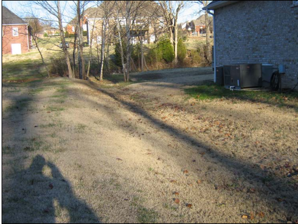
Item 9 – 407/409 Barnes Dr.. Grade ditch to drain into creek. Picture 2356.
