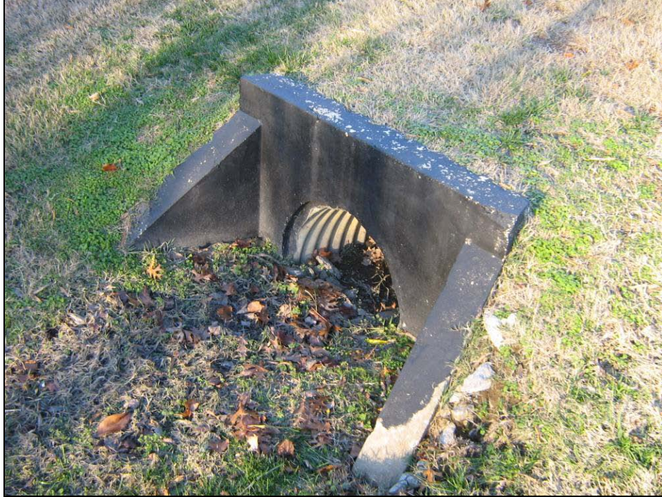
Item 7 - Lexington Dr. at Brunswick Dr. Clean out silt at outlet of 18" CMP. Picture 2370.
