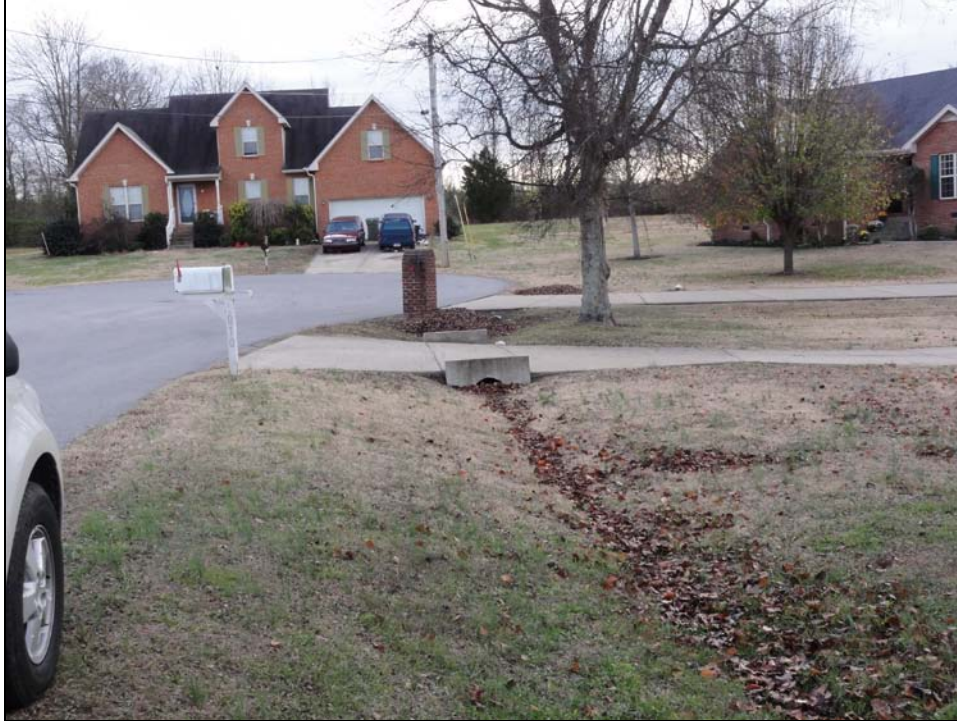
Item 7 – 1010 Jacquelin Dr. Clear debris and sediment from driveway culvert. Picture 1840.
