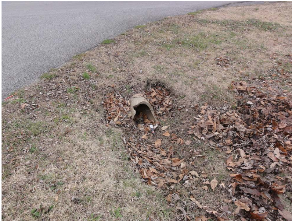
Item 3 – 421 Oakdale Dr. Repair damaged end of 6” VCP driveway culvert. Picture 1808.
