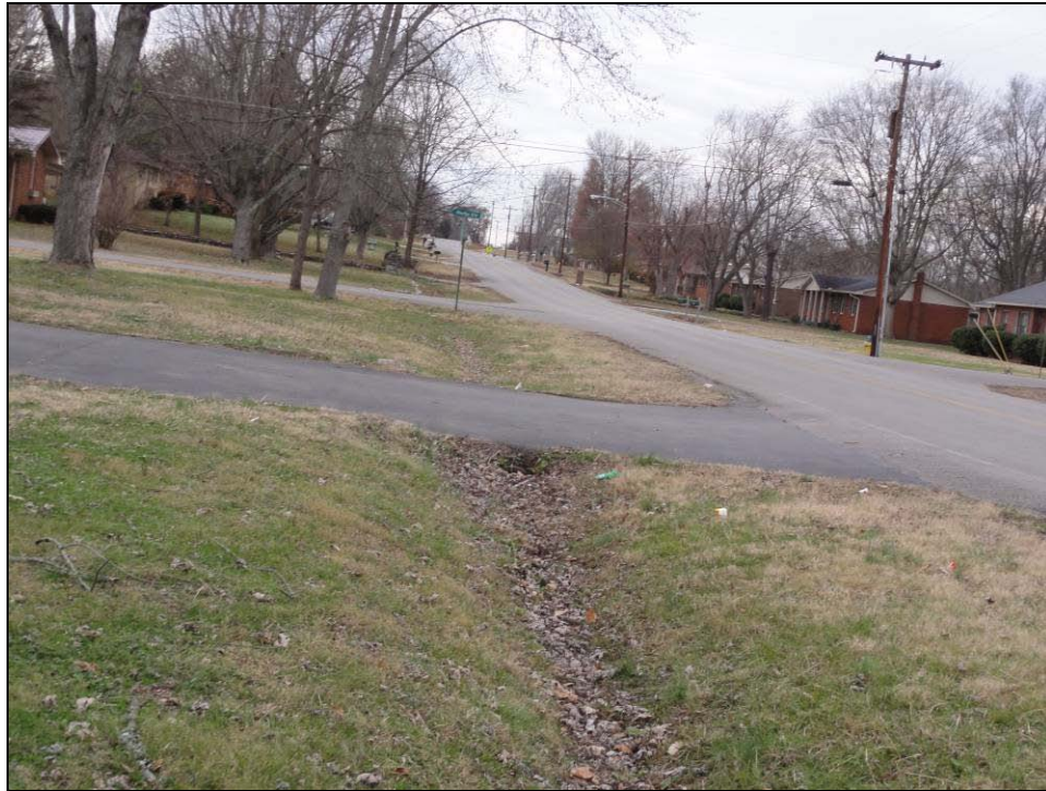
Item 1 – 107 Marks Cir. Clear debris from driveway culvert. Culvert is located on Oakdale Dr. Picture 1797.
