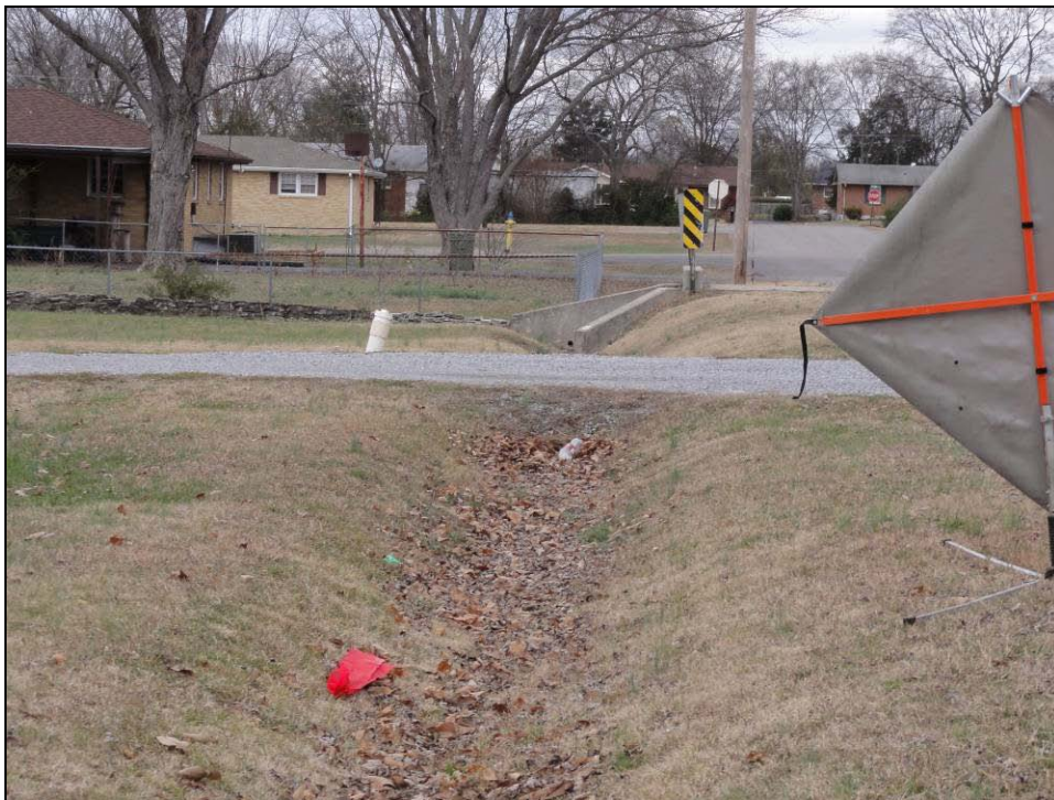
Item 4 – 417 Oakdale Dr. Clear debris and sediment from driveway culvert adjacent to Marks Cir. Picture 1809.
