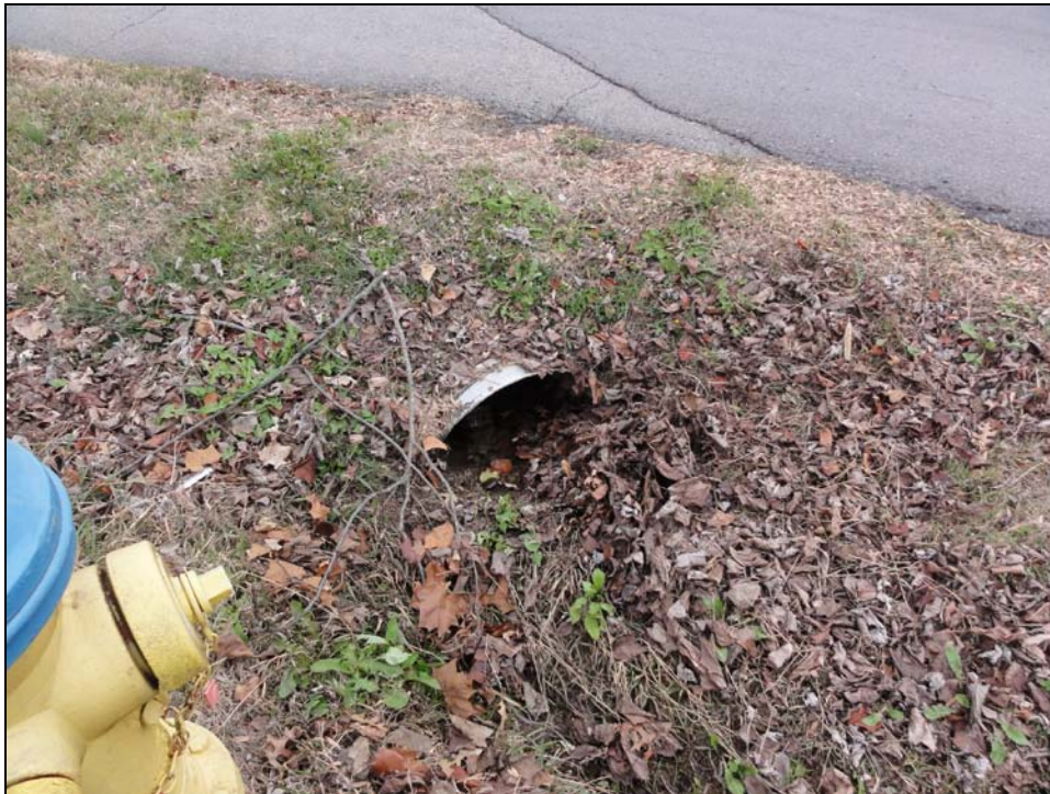
Item 6 – Lealand Ln. and Knoll Ln. Clear debris and sediment from 24” x 12” elliptical CMP. Picture 1840.
