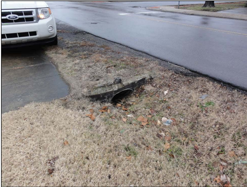
Item 1 W. Spring St. and S. Greenwood St. Clear sediment from 16" x 10" ellip. CMP. Picture 2167.
