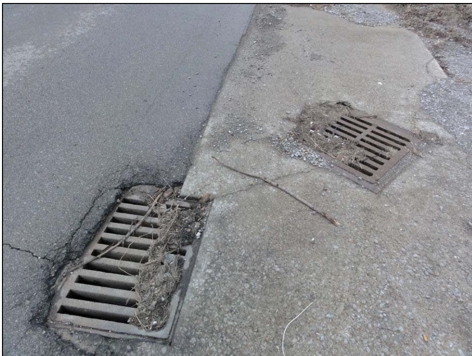
Item 26 – 319 S. Maple St. Clear debris from catch basin grates. Picture 2271.
