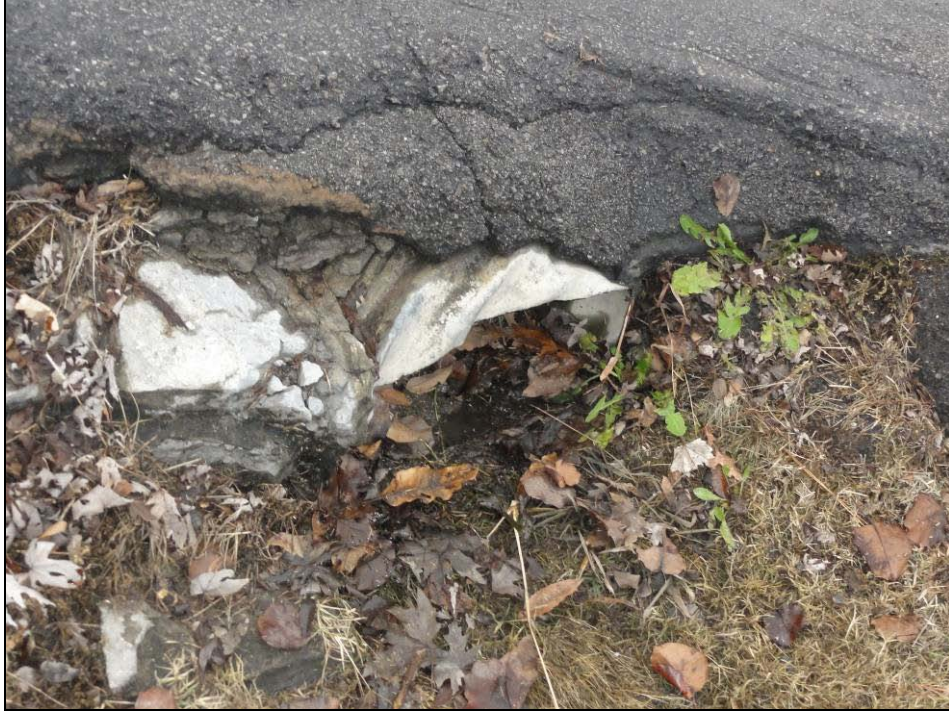
Item 33 – S. Tarver Ave. and McClain Ave. Clear sediment and debris from both ends 20” x 10” ellip. CMP cross drain. Repair end section. Picture 2315.
