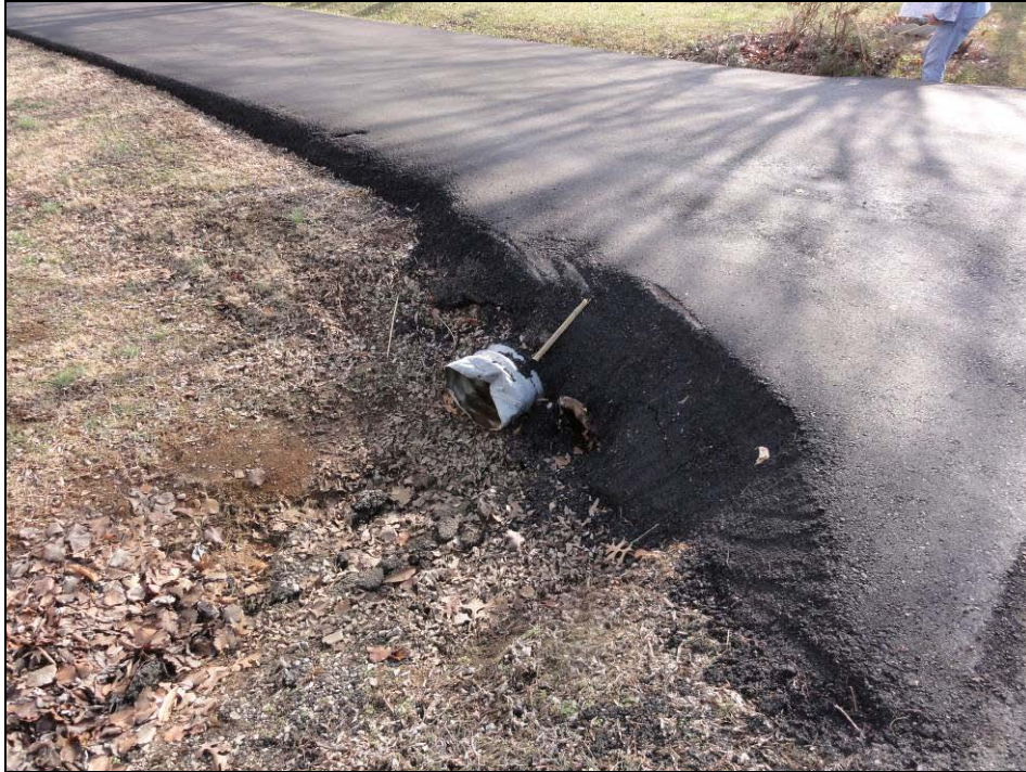
Item 50 - E. Sunset Dr. at S. Tarver Lane, west bound lane. Clear debris and sediment, repair damaged end sections of 2 – 14" x 10" ellip. CMP's. Picture 2414.
