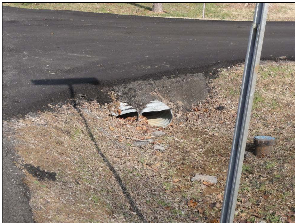
Item 49 – E. Sunset Dr. at S. Tarver Lane, east bound lane. Clear debris and sediment, repair damaged end sections of 2 – 14" x 10" ellip. CMP's. Picture 2413.
