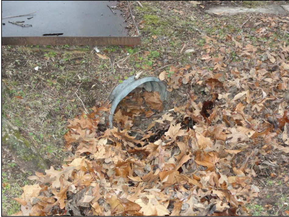
Item 19 – 514 W. Spring St. Clean debris and sediment from culvert inlet. Picture 2225.
