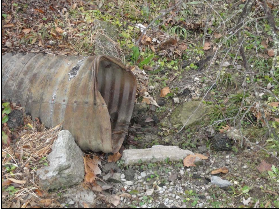
Item 37 – Martin Ave. and Cleveland Ave. Repair end of 26” x 20” ellip. CMP. Picture 2340.
