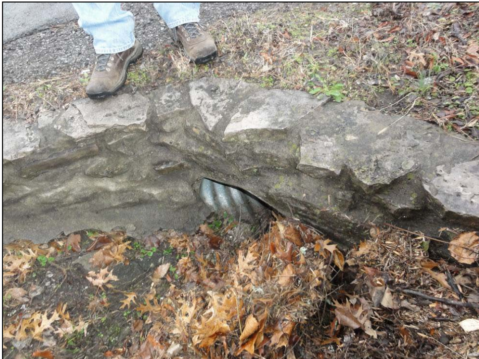
Item 22 – W. Spring St. and Pennsylvania Ave. Clear debris from west end of 15” CMP. Picture 2239.
