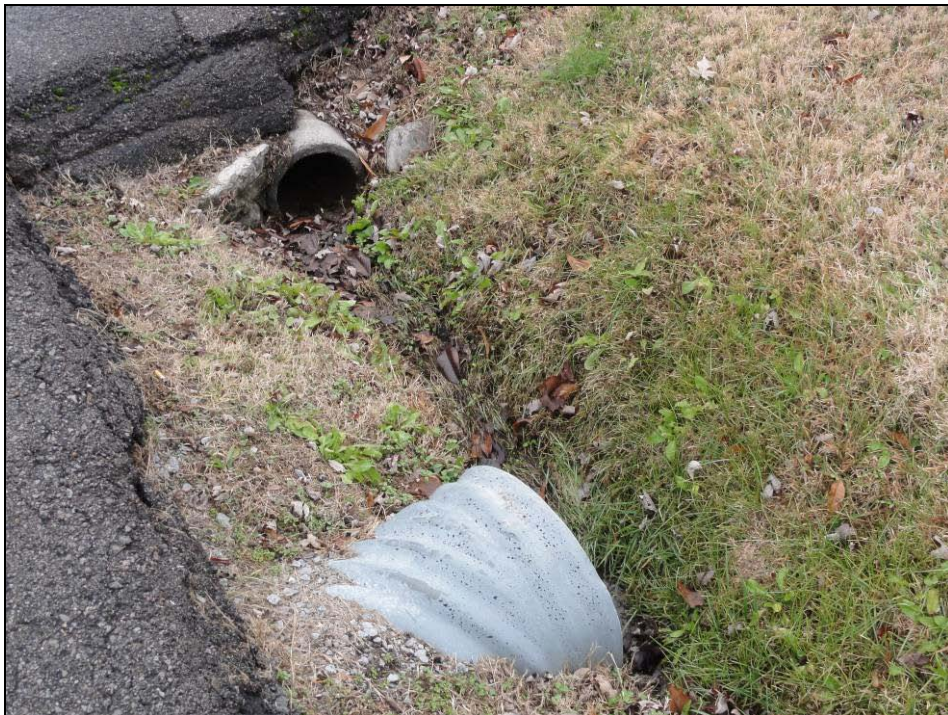
Item 47 – Pennsylvania and W. Sunset Dr. Improve ditch section at end of 18" CMP. Picture 2389.
