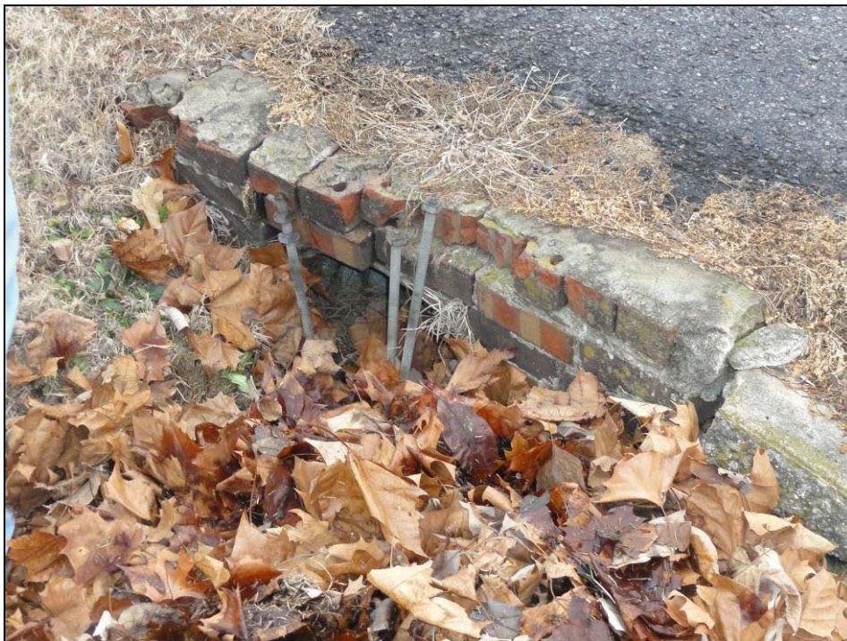
Item 2 - W. Spring St. and S. Greenwood St. Clear sediment and debris from 18" CMP. Picture 2169.
