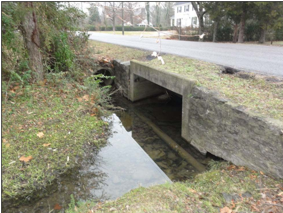
Item 20 – 514 W. Spring St. Improve channel section immediately upstream of 10' x 4' RCB. Picture 2230.
