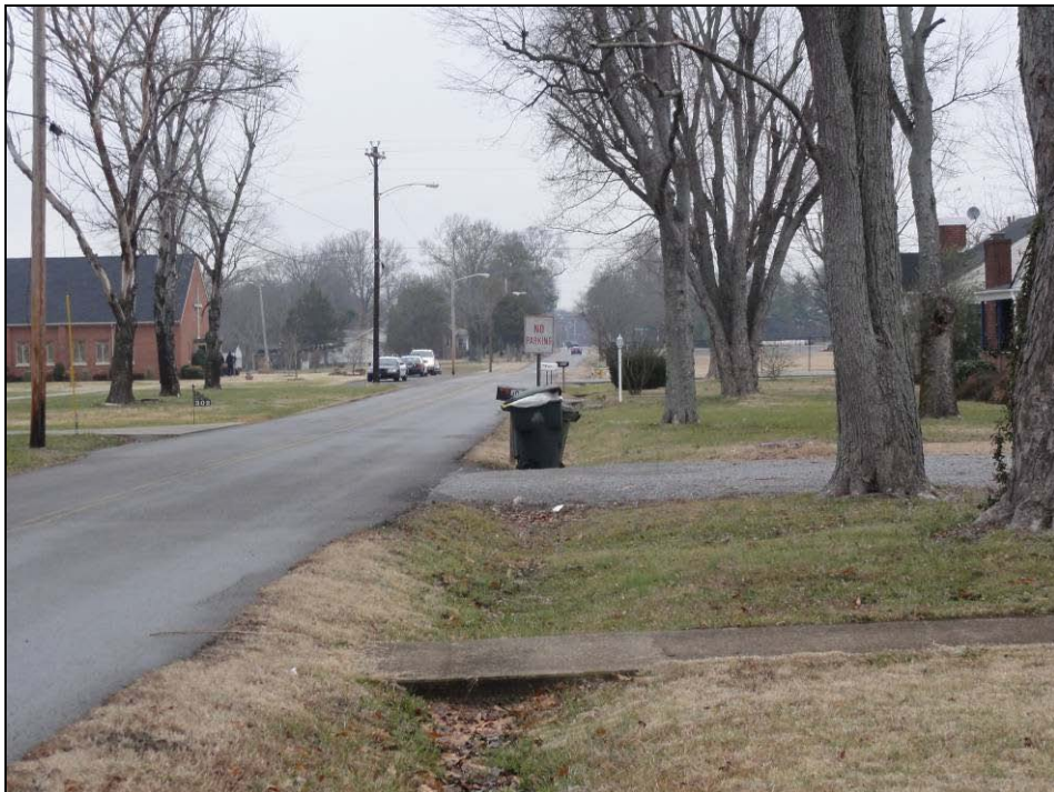
Item 34 – S. Tarver Ave. from Martin Ave. to McClain Ave. View is looking north towards McClain Ave. No culverts under sidewalks and driveways on east side of S. Tarver Ave. Provide positive drainage in ditch. Approx. 310 LF. Picture 2324.
