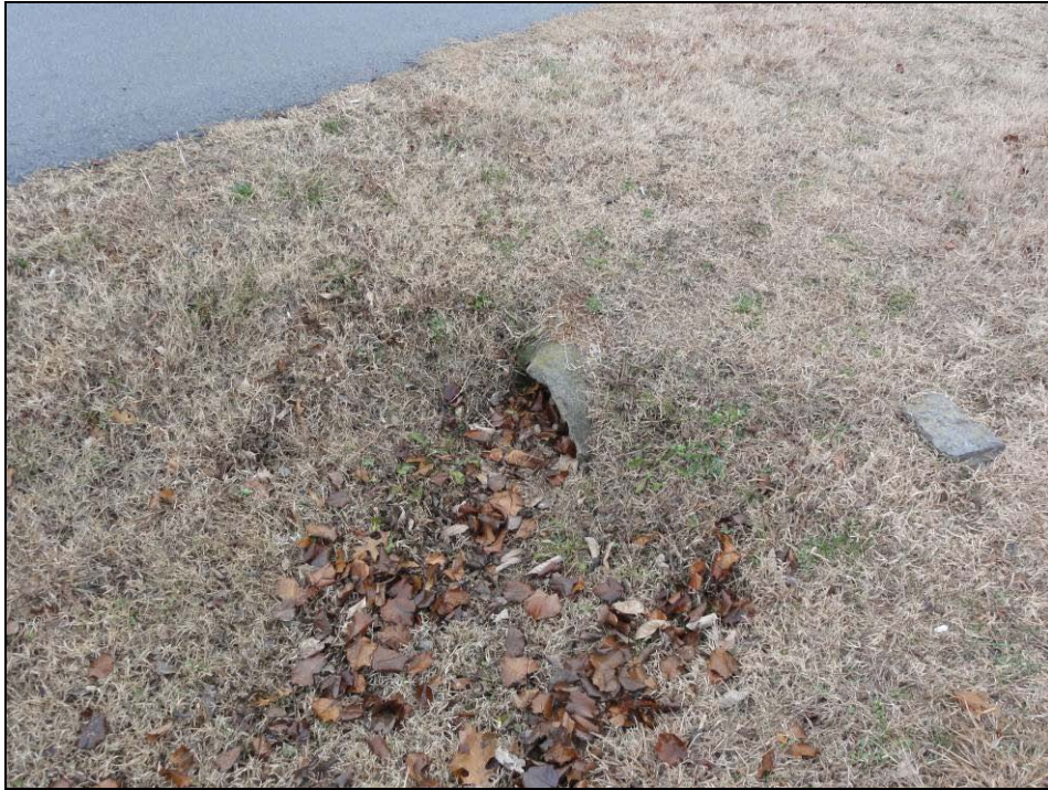
Item 7 – West side of S. Greenwood St. south of University Ave. Clear sediment and debris from RCP. Picture 2178.
