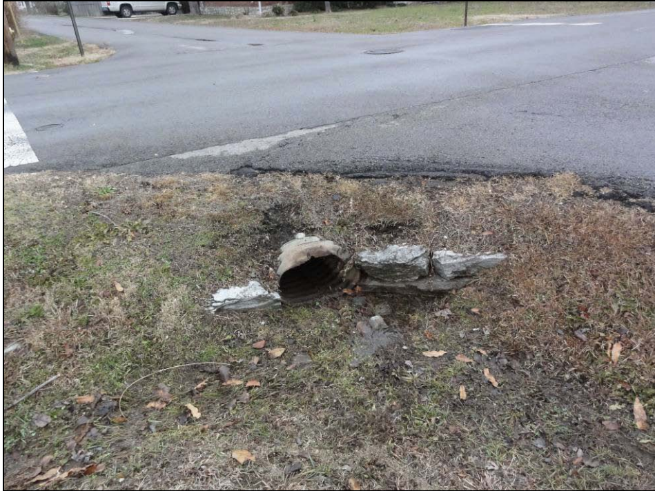
Item 35 – S. Tarver Ave. and McClain Ave. Repair end of 22” x 12” CMP. Picture 2326.
