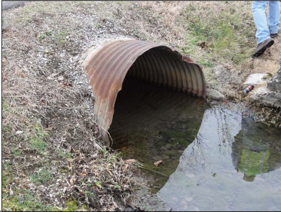
Item 46 - 511 W. Sunset Dr. Clear debris and sediment from 57" x 36" ellip. CMP. Picture 2380.
