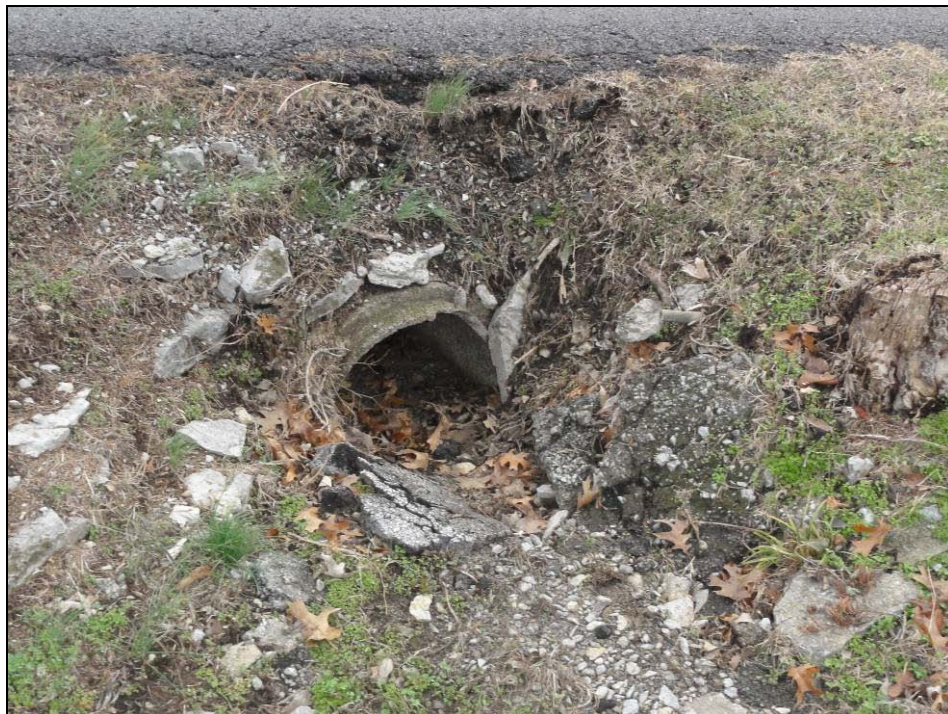
Item 30 – 224 S. Tarver Ave. Clear debris and sediment from both ends of 18” RCP cross drain. Picture 2305.
