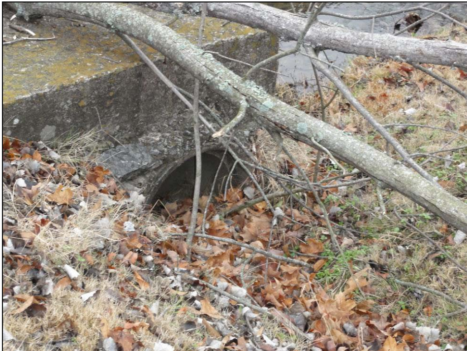
Item 36 – 431 Martin Ave. Clear debris from 15” RCP. Picture 2331.
