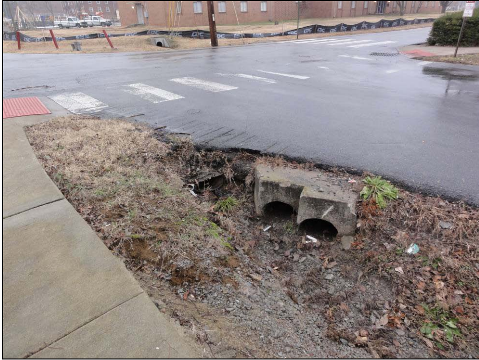
Item 10 – S. Greenwood St. and McClain Ave. Repair damaged end section of 12” CMP. Picture 2191.
