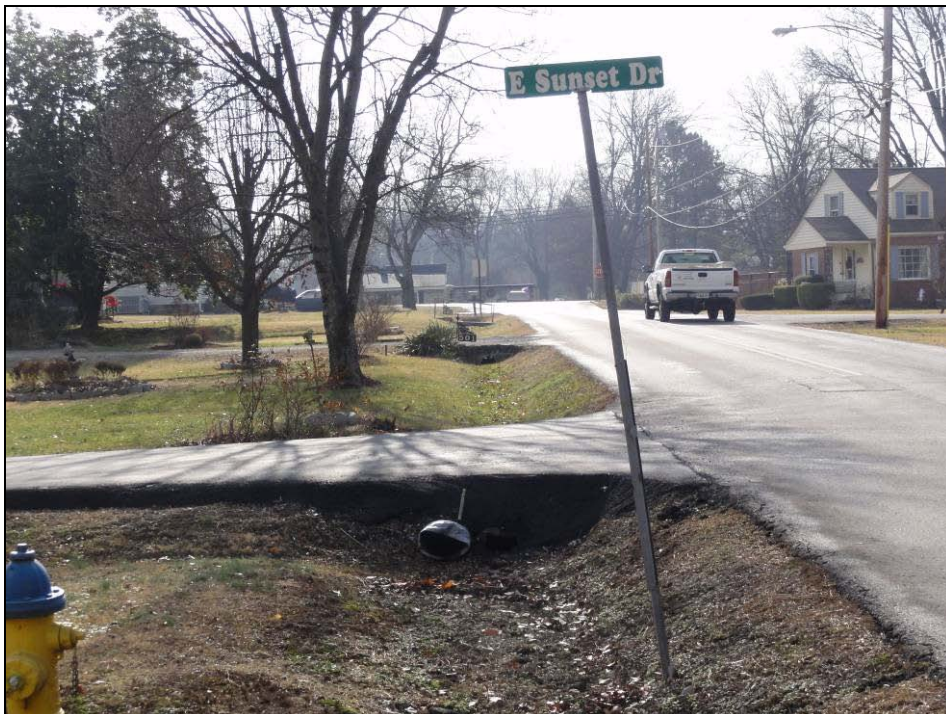
Item 51 – S. Tarver Ave from E. Sunset Dr. to Leeville Pk. View is looking south from E. Sunset Dr. Repair end sections of all driveway culverts. Picture 2411.
