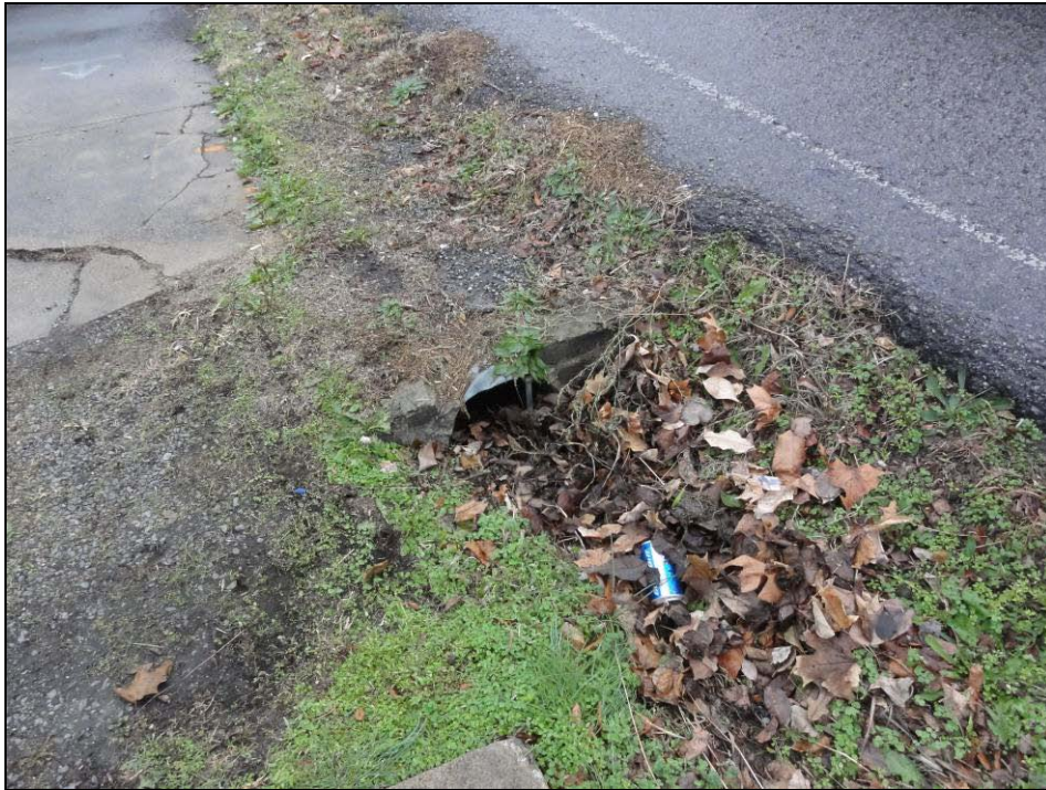
Item 3 – W. Spring St. and S. Greenwood St. Remove debris from 12” CMP. Picture 2171.
