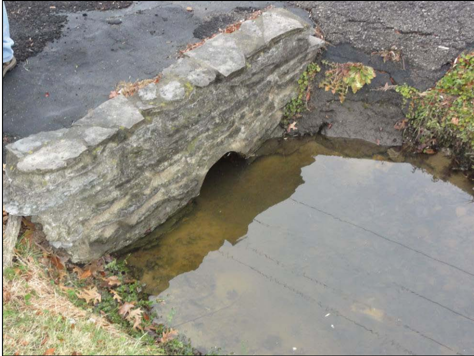
Item 23 – 520 W. Spring St. 24” CMP clogged with debris and sediment. Flush pipe and remove debris from ditch. Picture 2235
