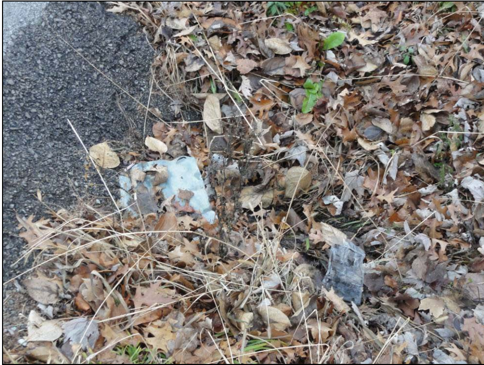
Item 42 – Wagoner St. and Pennsylvania Ave. Clear debris from 15" x 10" ellip. CMP. Picture 2352.
