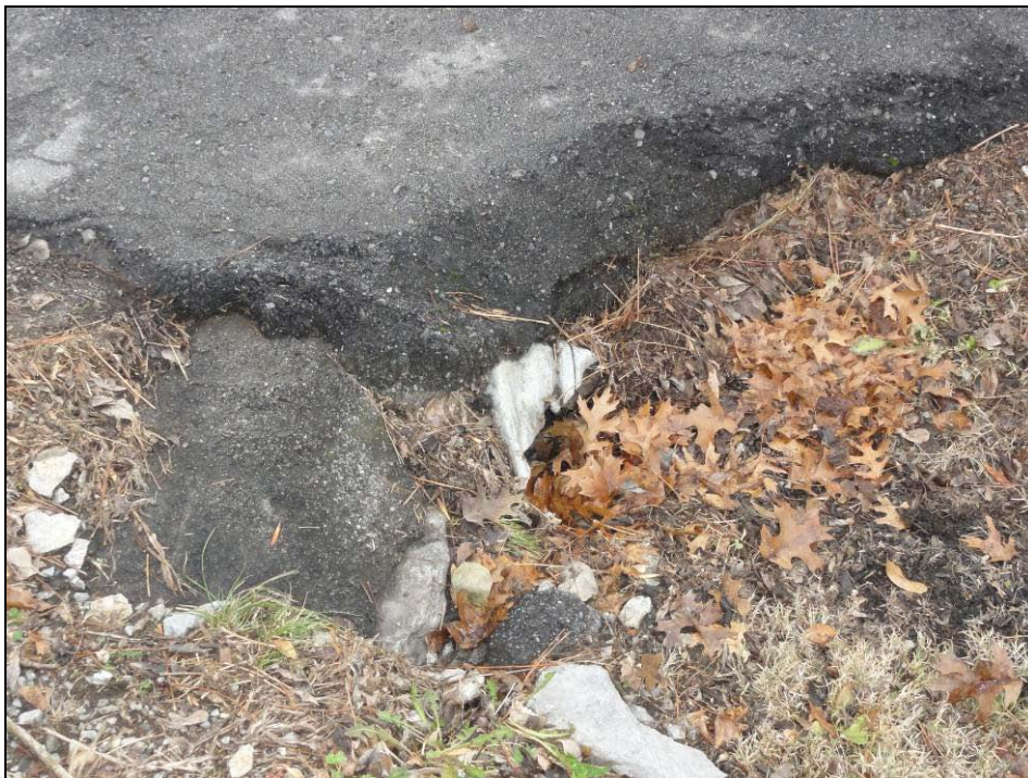
Item 28 – East side of S. Tarver Ave. Clear debris and repair end section of 12" CMP. Picture 2299.
