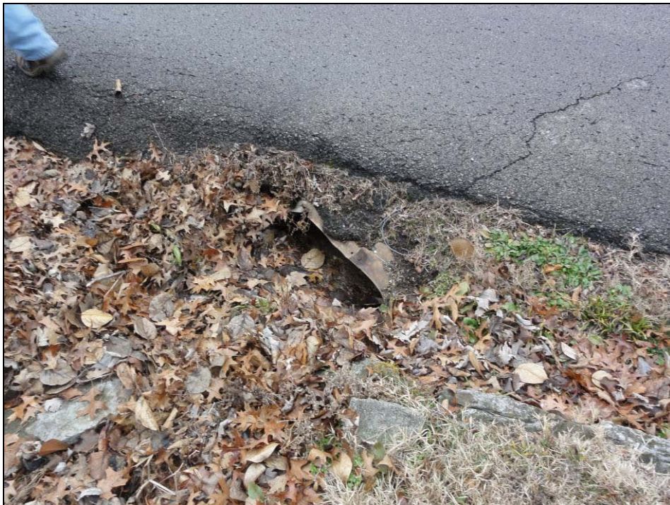
Item 40 – Cleveland Ave. and McClain Ave. Clear debris and sediment from 14" x 9" ellip. CMP cross drain and repair damaged end section. Note crack in pavement. Picture 2346.
