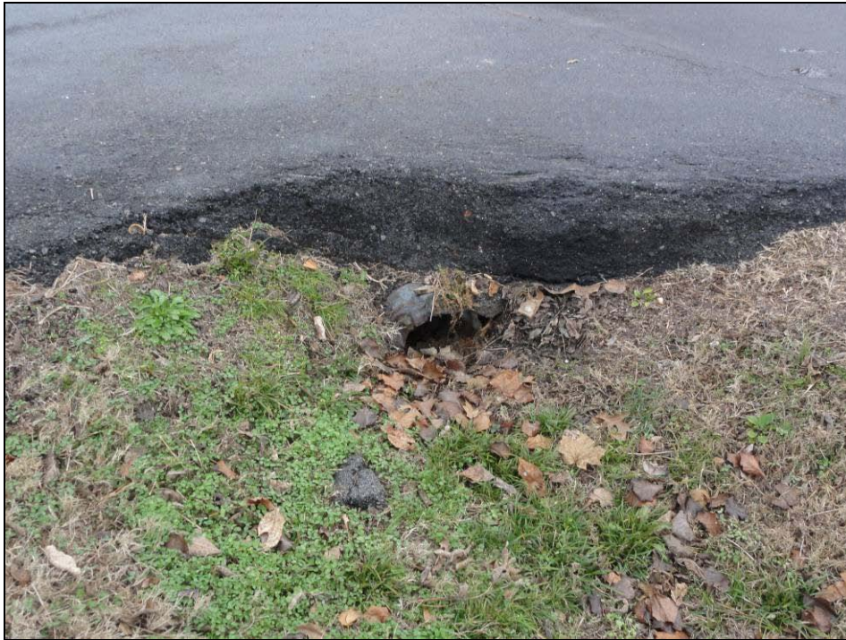
Item 5 – West side of S. Greenwood St. just north of University Ave. Clear sediment and debris from 12" CMP under parking lot access drive. Picture 2176.
