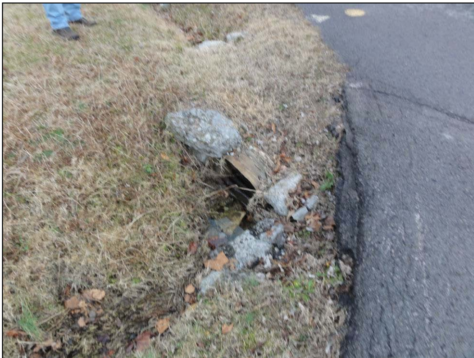
Item 43 – Martin Ave. and Pennsylvania Ave. Clear debris and sediment from 23" x 12" CMP. Picture 2356.
