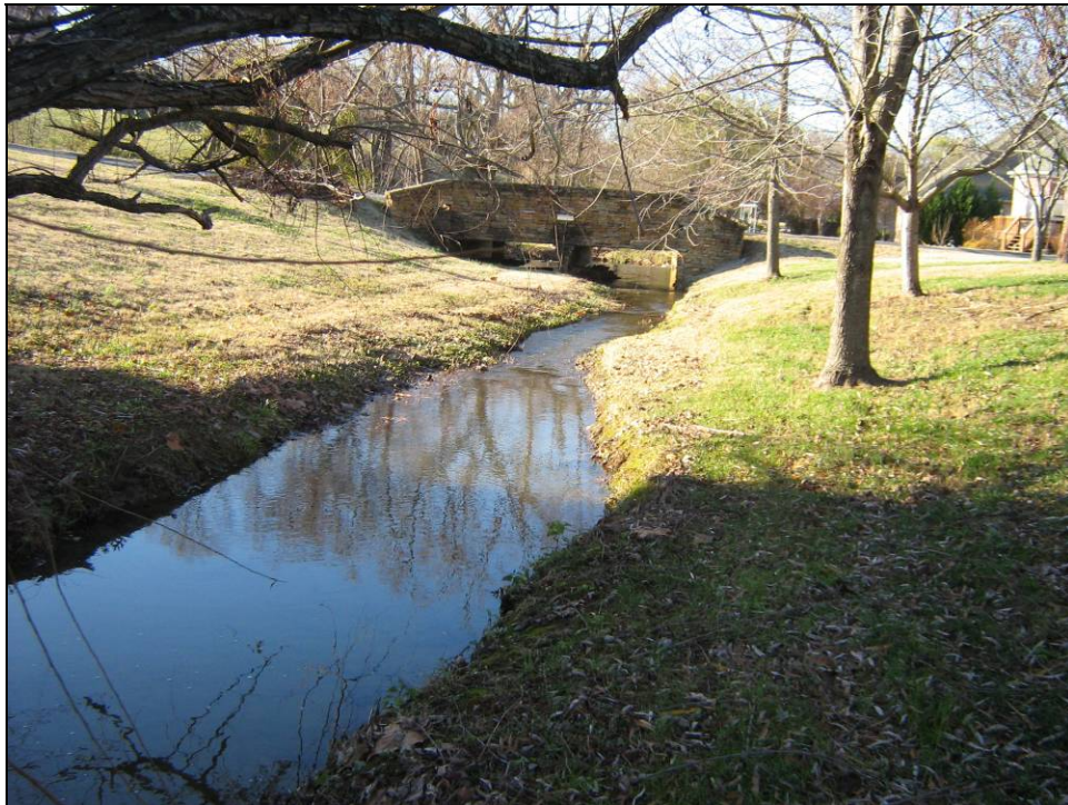
Item 2 – Looking north at Letcher Ave. Clear sediment from west span of double 8' x 3' RCB. Picture 2318.
