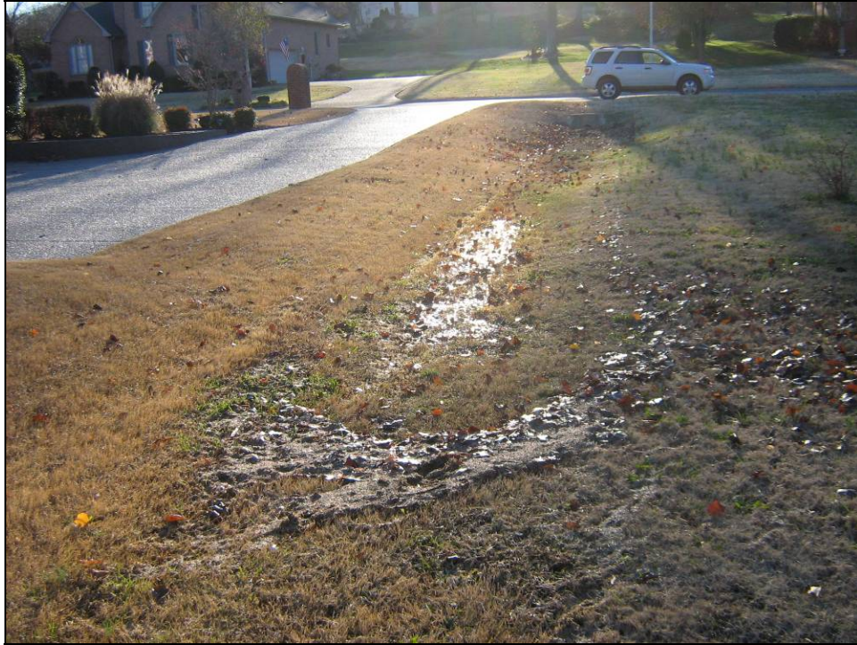
Item 5 – 409 Barnes Drive. Grade ditch to drain into creek. Looking upstream (west) toward Barnes Drive. Note standing water and debris. Picture 2352.
