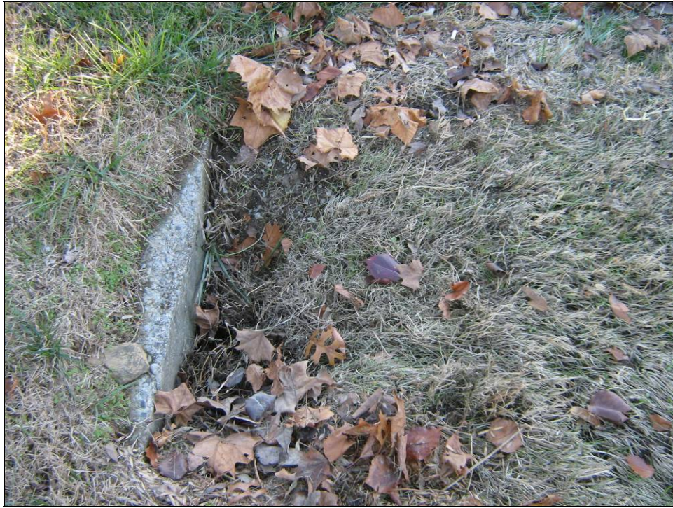
Item 1 - 18" RCP on Lexington Dr. north of Vicksburg Ln. Clear debris and sediment from 18" RCP culvert. Picture 2312.
