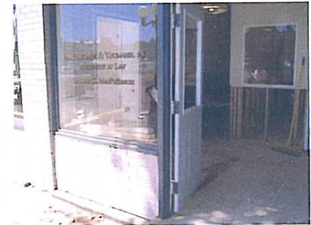
This picture also from the Town Square, signs of the beginning of repair to flood damaged areas.
