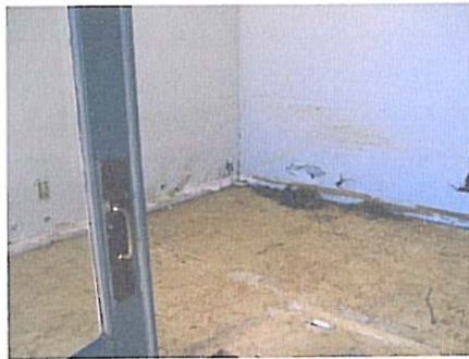
Evidence of flood damage in an office on the Town Square.
